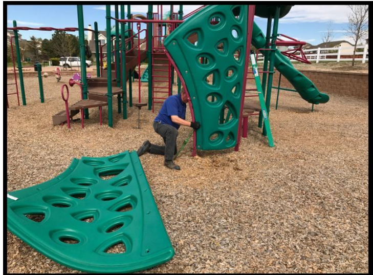
District Team Member Dana Stern replacing climbing wall in children's play area in South Manchester Park.
